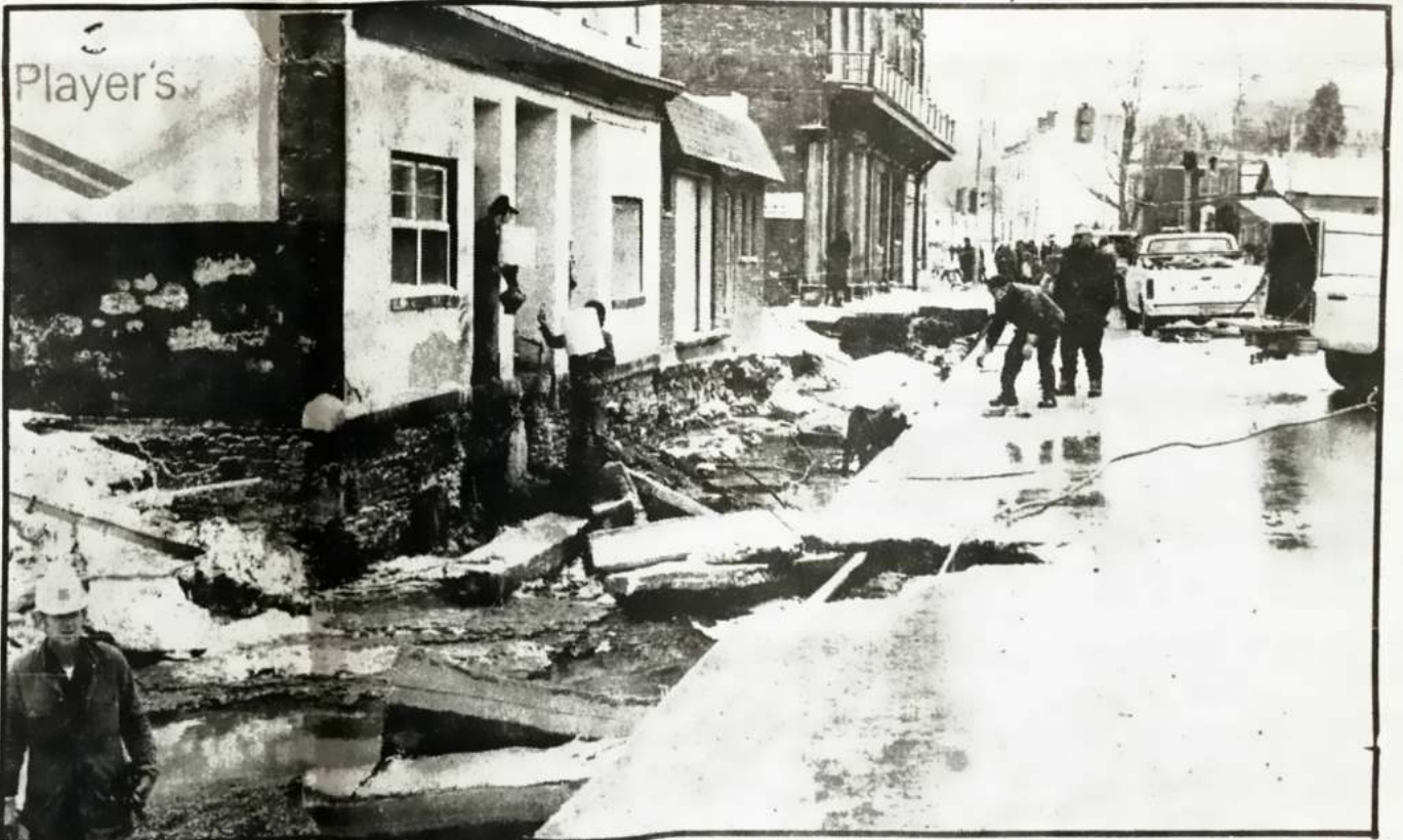
The scene on Mill Street just below Walton Street, Saturday morning. Residents returned to salvage their personal belongings as road crews checked an exposed gas line.
